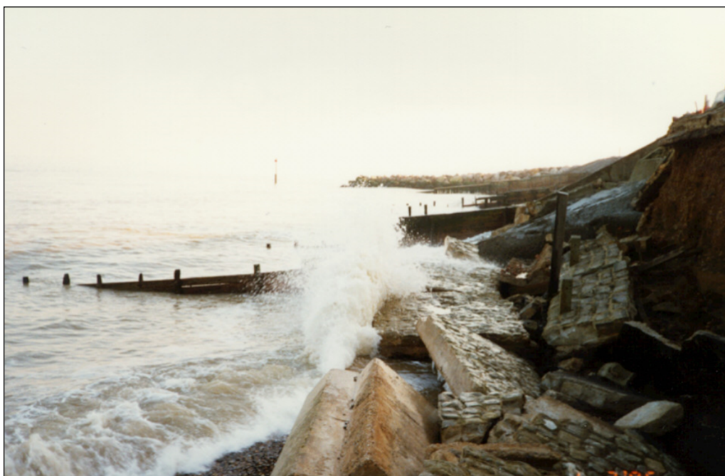
Figure 5.4 - Failed Seawall at Reculver caused by the 1996 Storm
